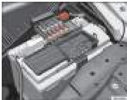
Fig. 140 Fuse box above battery
