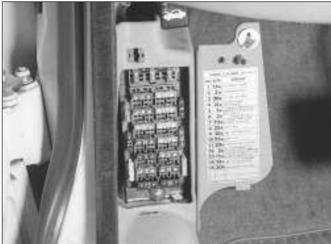
3.1a The left side fusebox is located in the passenger's side kick panel, behind the fuse panel cover
