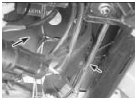
10.7 Remove this brace rod (small arrow) for clearance to remove the left blower motor housing (large arrow)
