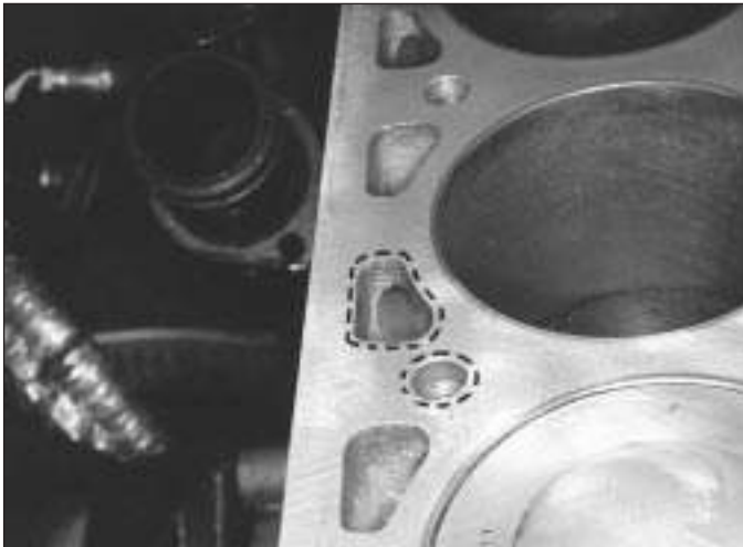
10.12 Place the new head gasket on the engine block, and trace around the water passages and bolt holes - make sure there is no erosion of the aluminium beyond these lines
