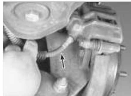
11.11 Check along the brake hoses and at each fitting (arrowed) for deterioration and cracks
