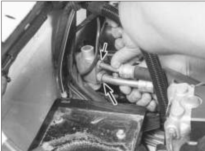
13.9 Feel the inlet (small arrow) and outlet (large arrow) pipes at the bulkhead leading to the air conditioning evaporator (battery removed here for clarity only)
