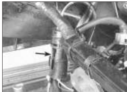
15.4a Disconnect the solenoid electrical connector at the harness connector located near the bulkhead behind the cylinder head (arrowed)
