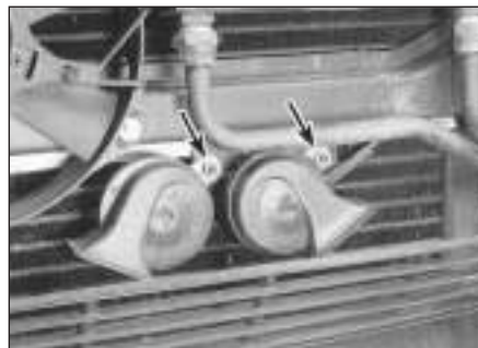
20.9 Disconnect the electrical connector, remove the retaining nuts (arrowed) - then detach the horn(s)
