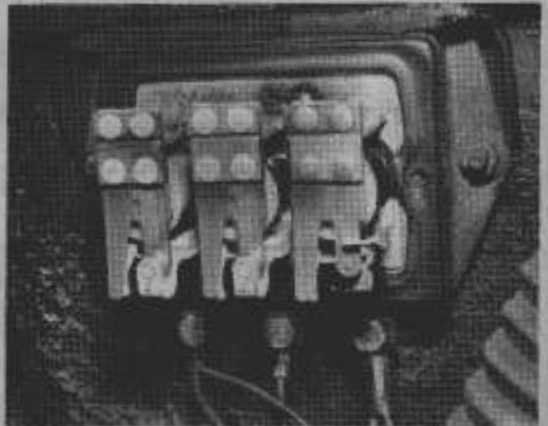
Fig. 8.8. As you look at it, voltage regulator on the left (above terminal 51), current control in the centre, and cut-out right (above terminal 30).
