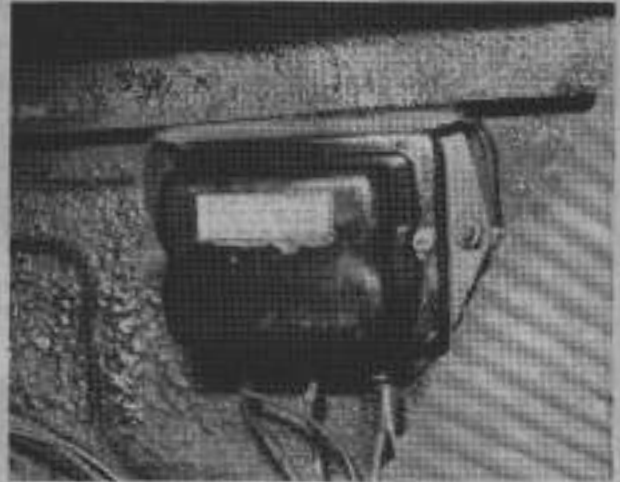
Fig. 8.7. The control box showing the terminal numbering
