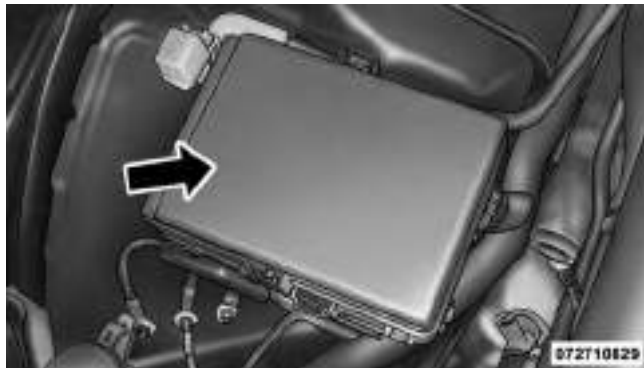
Front Power Distribution Center
