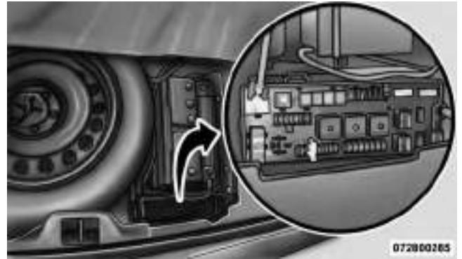
Rear Power Distribution Center
