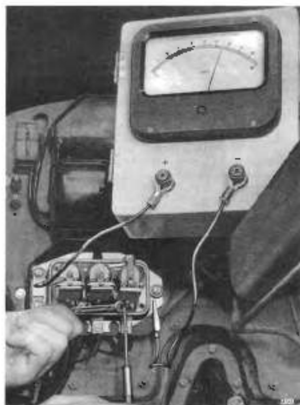
Fig. M14 Cut-in voltage adjustment
