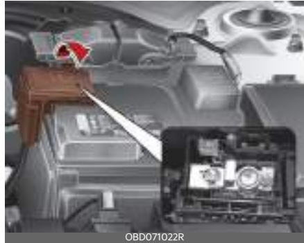
Engine compartment fuse panel (Battery terminal cover)
