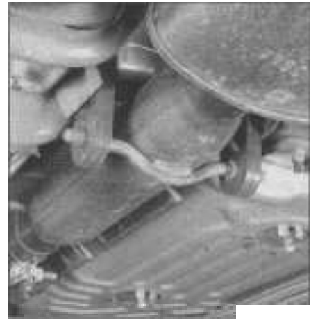
18.1 Inspect the exhaust system mounting brackets, clamps and rubber hangers for damage or improper installation
