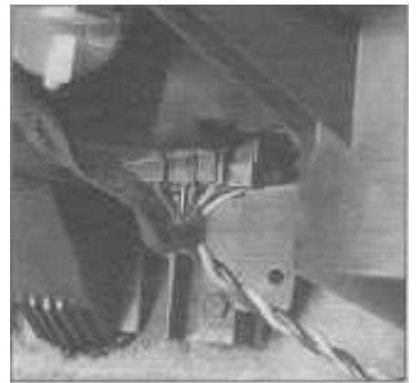
9.3 Using suitable probes, backprobe the blower harness plug (twisted pair of wires) at the blower motor resistor block - connect a voltmeter to the dark blue wire (+) and black wire (-), voltage should vary as the blower switch is moved through each position
