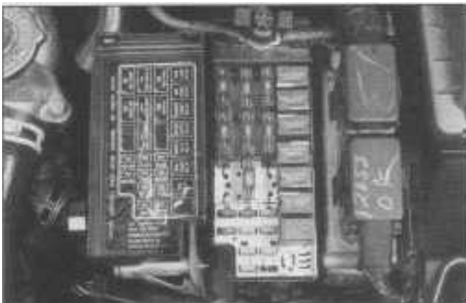
3.1b The Power Distribution Center is located in the engine compartment and contains both fuses and relays (additional relays are under the square cover directly above the PDC)
