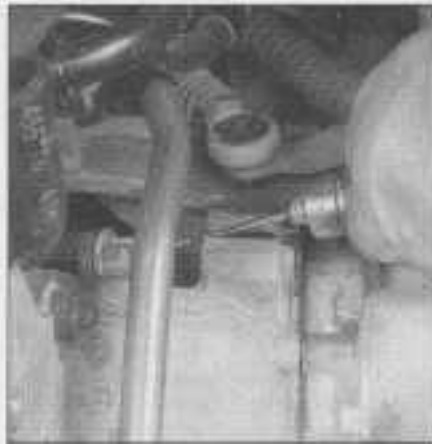
3.4 Grab onto the clutch cable housing, pull it back and pass the clutch cable through the slot in the bellhousing, then disconnect it from the release lever
