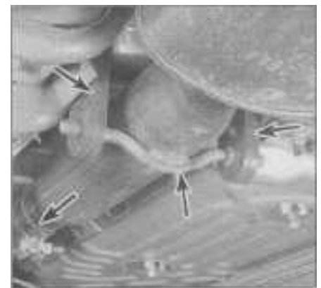
15.3 Check the exhaust system connections, clamps, mounting bolts, brackets and hangers for damage (arrows)
