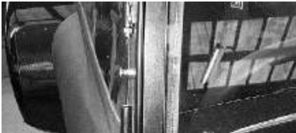
Figure 212: Stud located on stanchion
