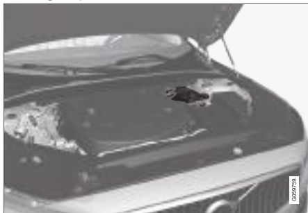
The 12 V support battery is located in a box next to the strut tower.
