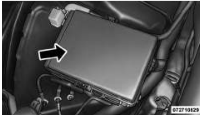
Front Power Distribution Center
