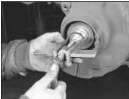
8.8b If the inner race of the bearing sticks to the stub axle, use a puller to get it off
