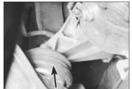
17.4 As engine mountings wear or age, they should be inspected for cracking or separation from their metal plates
