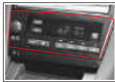
Air conditioner control panel
